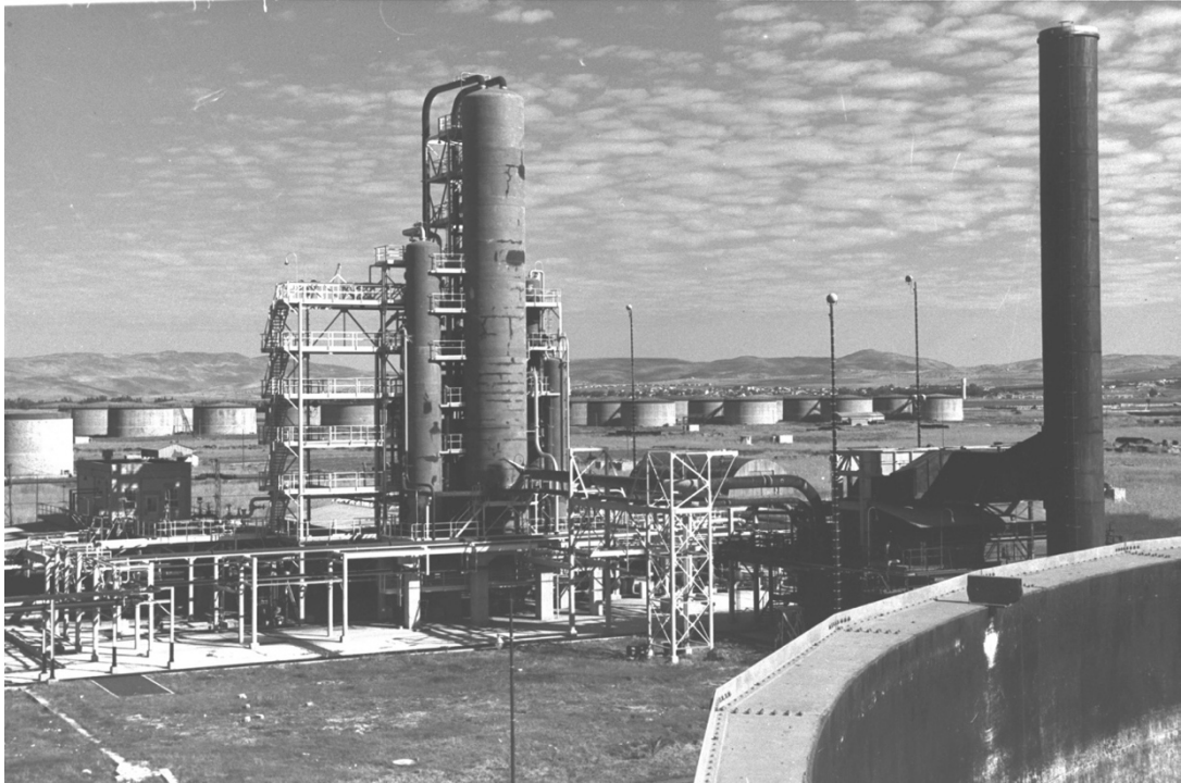
Crude oil tanks and towers at the Haifa oil refineries, 17 December 1950. Photo Credit: Cohen Fritz, Israeli Government Press Office.
