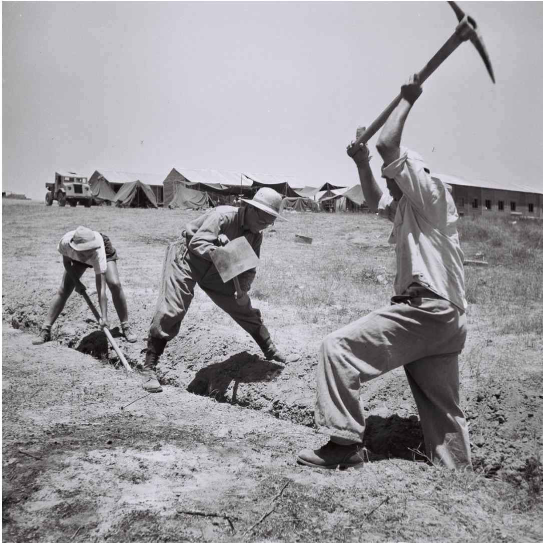
"Mekorot" Workers Laying a Waterpipe Near Kibbutz Mefalsim in the Northern Negev, 6 July 1949. Photo Credit: Kluger Zoltan, Israeli Government Press Office.
