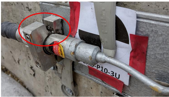
Figure 6 Destroyed screws of an earth pressure sensor.
