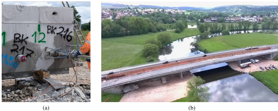
FIGURE 1. (a) Sampling of the drilling cores and (b) bird's eye view of the investigated bridge in Roding.
